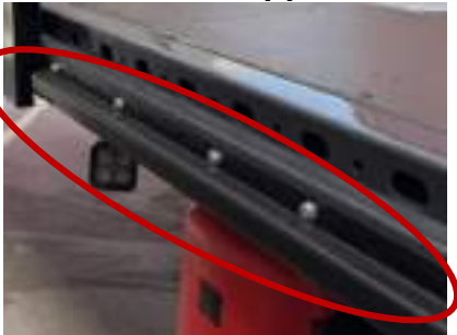
Steel forklift barrier
